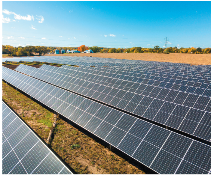
Tyto Solar in Fitchburg is a 6-MW solar project to serve all MGE customers.
